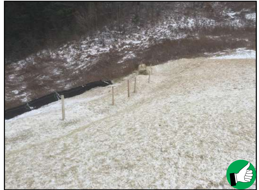
Stabilization and seeding of slopes before winter will reduce or eliminate erosion in the spring.
