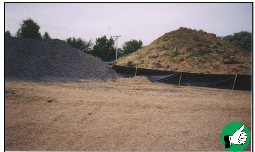
Excellent application of hay mulch. Good mulch cover and perimeter control around soil stockpile.
