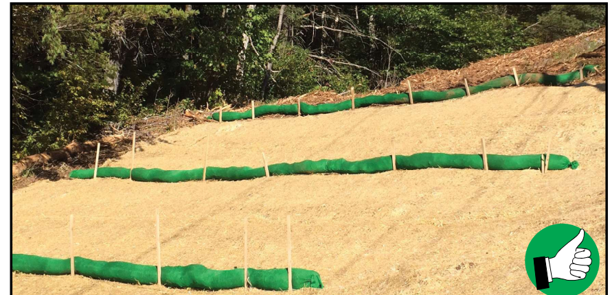
Good use of filter socks along a slope to slow runoff velocity.
