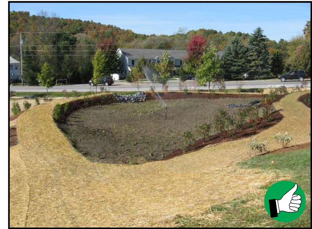
Infiltrating stormwater practices such as this bioretention system should be kept offline until the drainage area has been fully stabilized.
