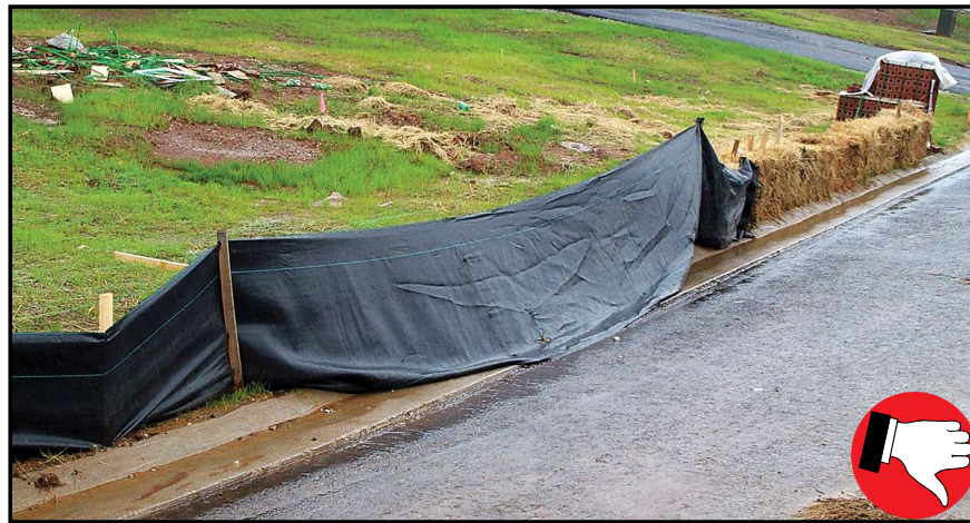
Poor installation of silt fencing. Silt fence must be trenched in along bottom. Hay bales are not approved as sediment barriers.
