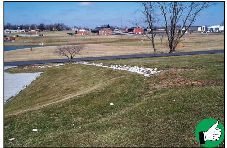
Good construction, seeding, and stabilization of diversion berm. Note that diversion ditch is lined with grass on flatter part of slope, and with rock on steeper part.
