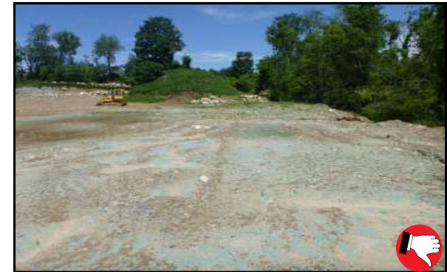
Poor hydroseed application. Not applied at the appropriate rate, soil not prepared, and very little mulch component in mix.
