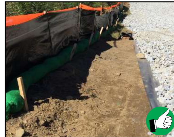
Use of a combination of silt fence and filter sock in place of reinforced silt fence for winter construction perimeter control requirements in proximity to a water resource area.
