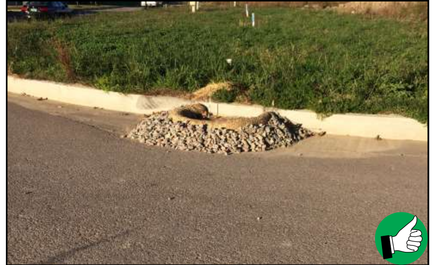
Use of stone inlet protection with the incorporation of a straw wattle in place of cinder blocks for the stone and block specification.
