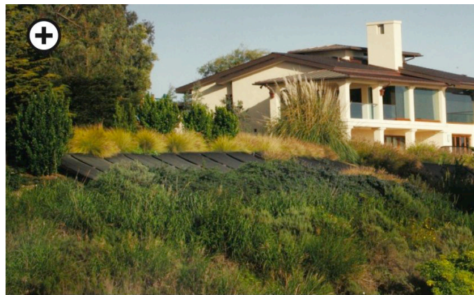
This ground-mounted array is well integrated into its site with native landscaping, making it less visible. From the City of Santa Barbara, Solar Energy System Design Guidelines (2006), p. 30.
