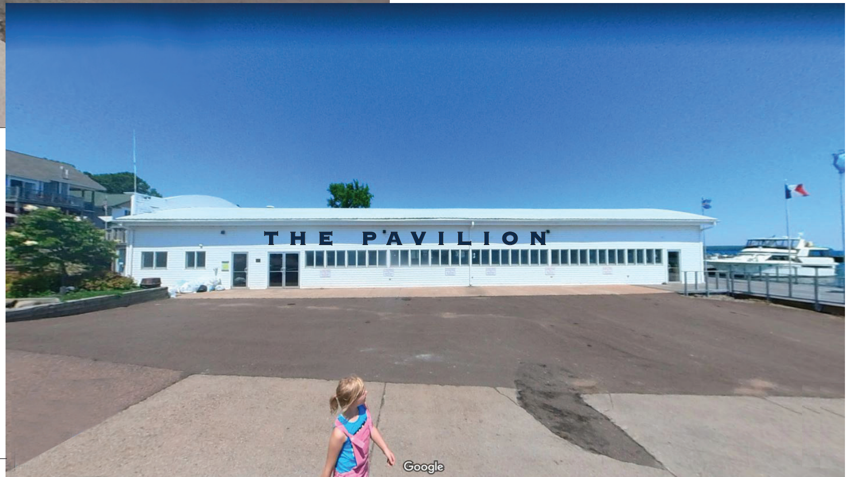
Painted letters cut out of material (acrylic, aluminum) and secured to wall.
